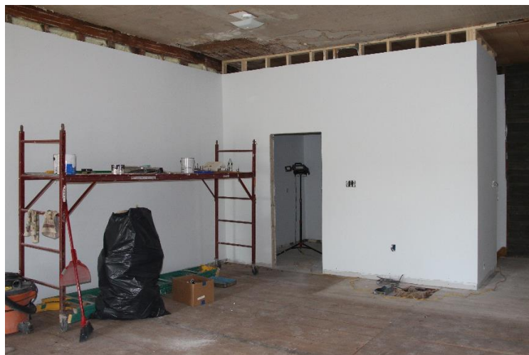
This photo was taken upstairs in Judd Hall from what will be the Nicholas Juried Museum of Jefferson History. The room through the doorway will be the Sally Swantz Archive Room. This original plank floor will be sanded and refinished. A dropped ceiling with simulated antique tin ceiling tiles will be installed at the upper edge of the dry wall
