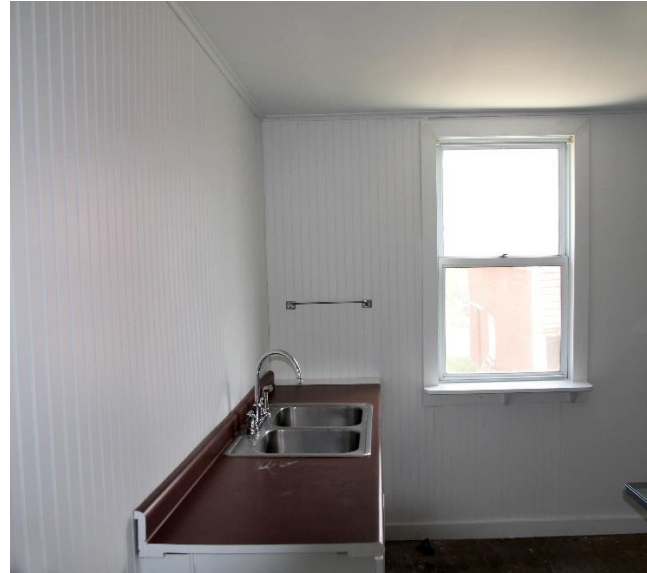
After: We removed the damaged areas of the wall and ceiling, insulated the wall, placed sheetrock on the ceiling, and paneled the wall behind the sink. Volunteers recently painted the kitchen walls, ceiling, and cabinets.
