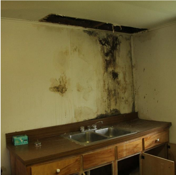
Before: The kitchen walls and ceiling were heavily water-damaged when we purchased the Masonic Hall.
