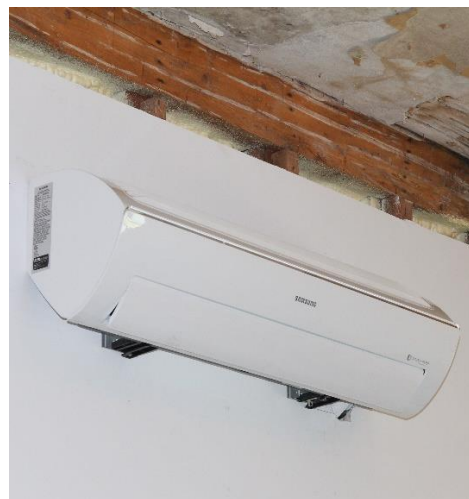
One of the two heat and air-conditioning units in the museum room.
